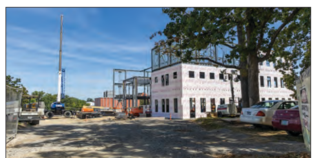
Jackson Hall construction taking place on the former faculty and staff parking beside Faculty Hall
