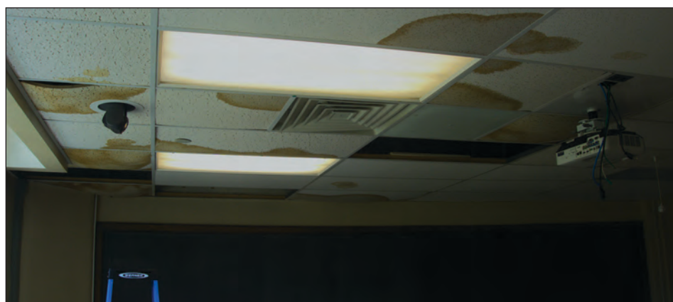
Top, Wilson Hall room 202 is tapped off from campus community. Middle, the classroom is shown after clean-up. Bottom, this shows the damage left behind from the leak.
