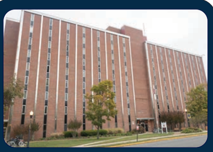
Photo courtesy of murraystate.edu The water pipe burst in RH White College causing damage to the east end of the building.
