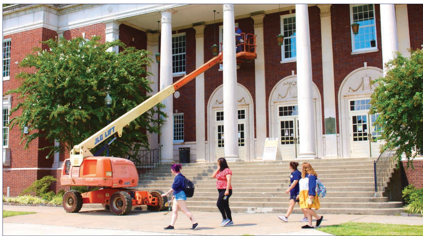
Lovett auditorium is set for a grand opening in October 2022, after being under construction since Spring 2021.
